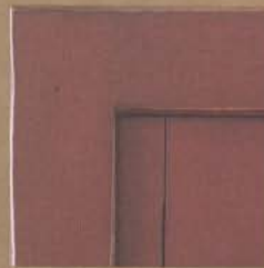
Light Distress & Oversand
